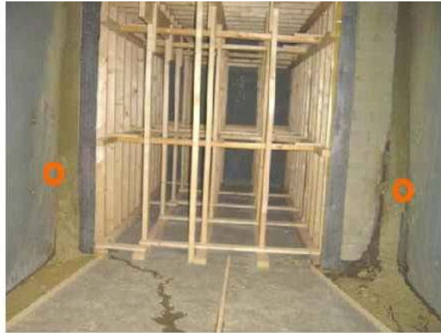
Inflow 0.25 l/min left, 0.5 l/m right Test duration 168 h, Initial outflow @ 24 h
