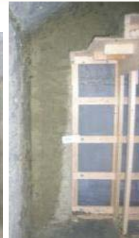
Extensive wetting behind inner fracture
