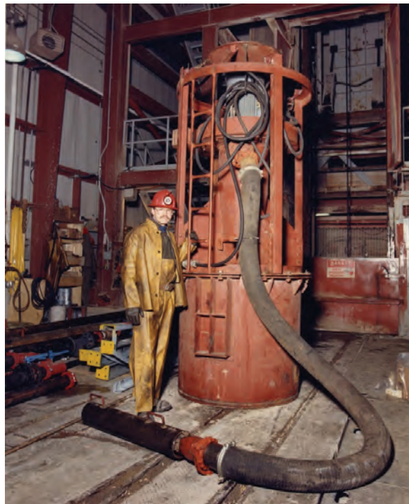
Figure 8: Vacuum Unit for Shaft Bottom Cleaning
