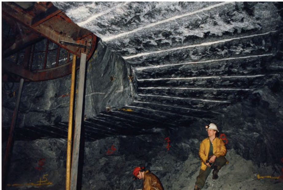
Figure 14: Controlled Drilling and Blasting Use to Provide Smooth Rock Surface for Geological Mapping
