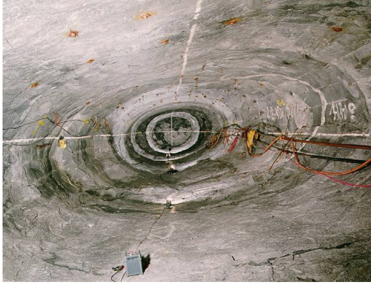
Figure 12: Stable Inclined Drill-and-Blast Tunnel from the Excavation Stability Study (Read and Chandler, 1997)
