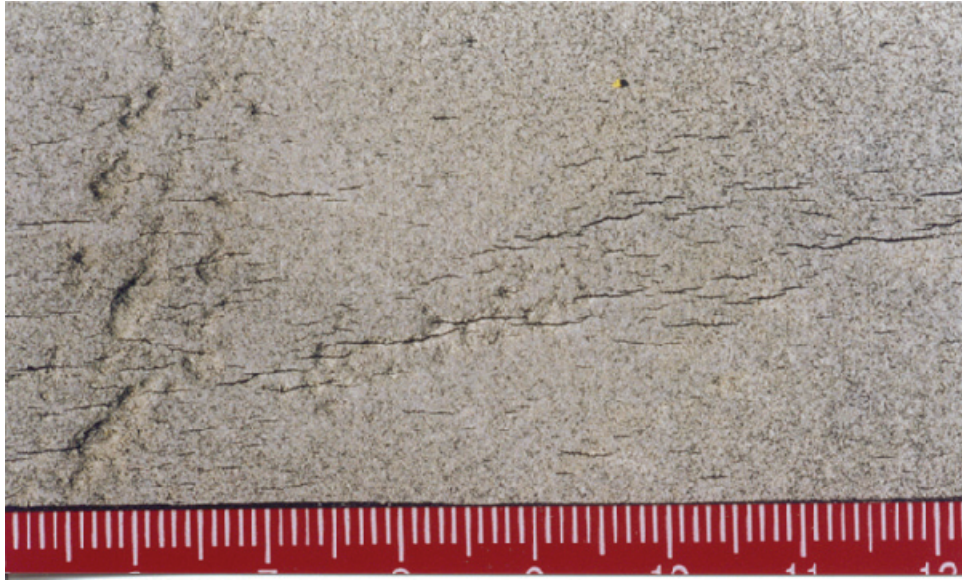
(a) Surface appearance of near-neutral pH SCC cracks on a cleaned pipeline surface
