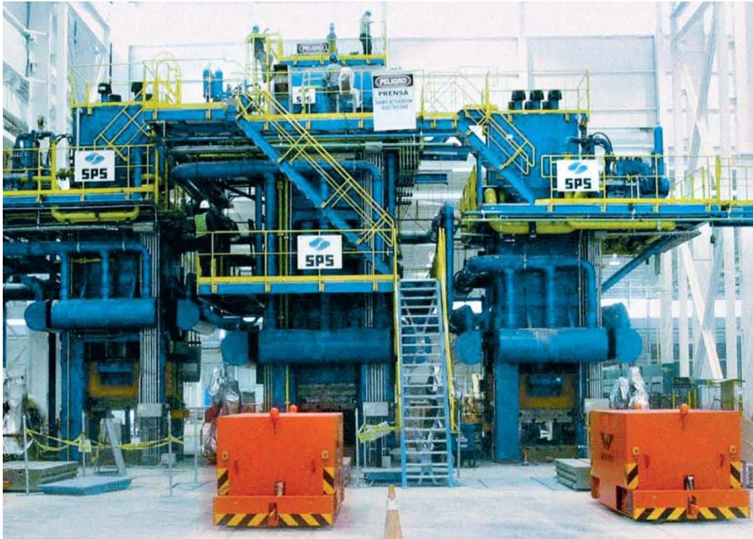
Figure 3-6: Example of a Large Press for the Sealing Materials Compaction Plant
