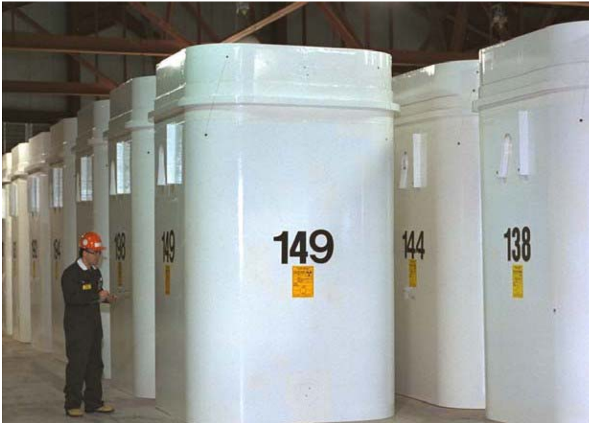
Figure D-6. Dry storage containers holding spent fuel inside the Phase I Building at Pickering NGS (OPG).
