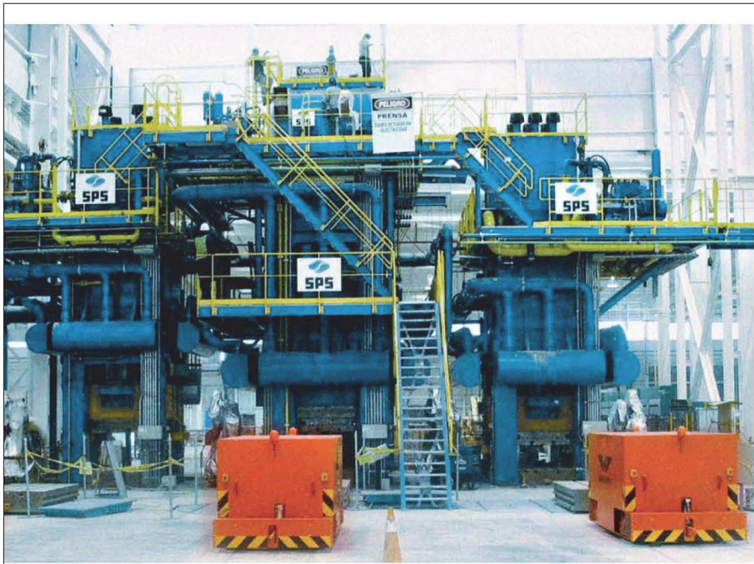
Figure 3-6: Example of a Large Press for the Sealing Materials Compaction Plant
