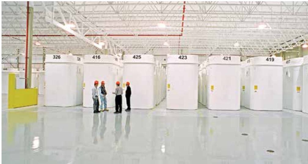
Ontario Power Generation used nuclear fuel dry storage facility
