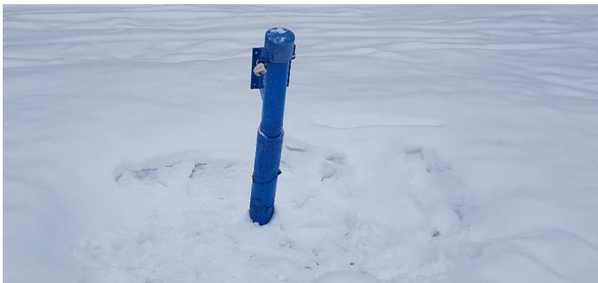
Figure 11: IG_BH03 Wellhead with protective casing and monopod bracket installed.
