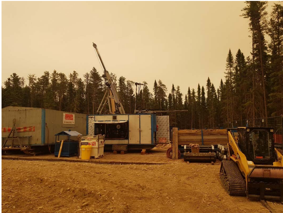
Photo 9: Facing east towards the drill pad. From the left are the drill water settlement tanks, auxiliary generator, fuel storage tank, drill rig, drill rod holders, and temporary skid steer.
