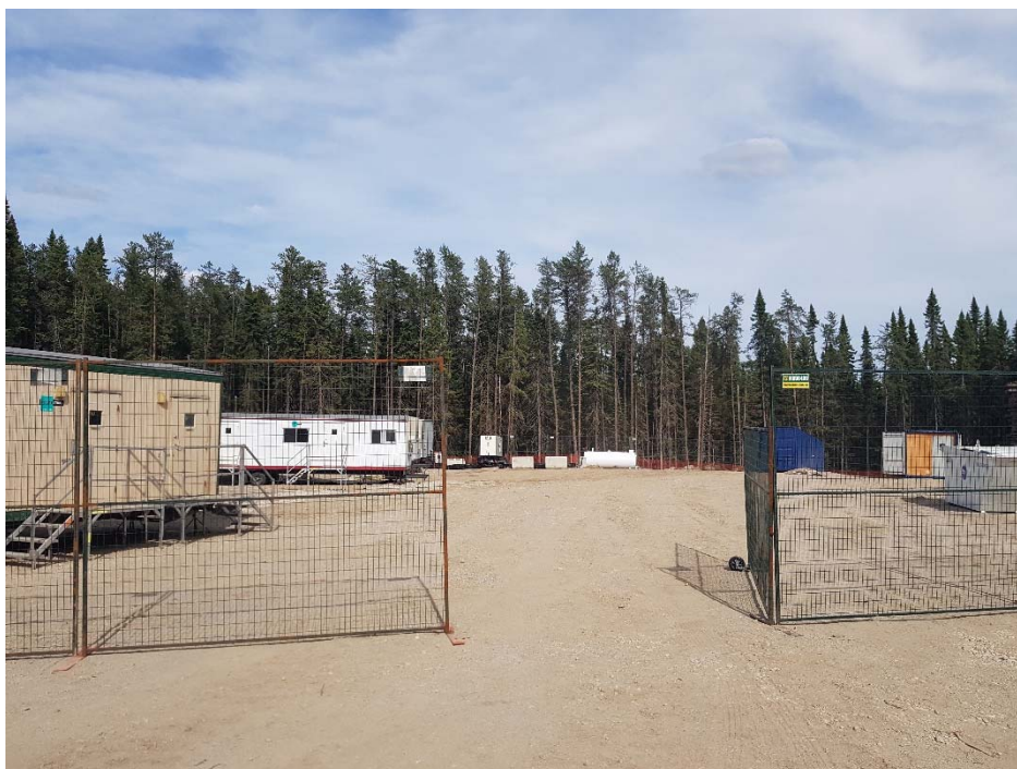
Photo 6: Facing East from the parking lot on June 27, 2019. Visible from the left are the wash cart, three office trailers, generator and fuel storage tank (not yet in place), core storage seacan, core logging seacan, garbage and recycling bins.
