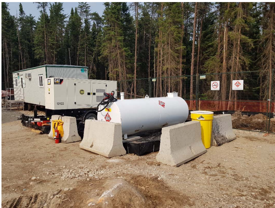
Photo 7: Facing north towards the site generator and fuel storage tank. Concrete barriers were placed around the fuel storage tank to protect it from inadvertent contact by heavy equipment.
