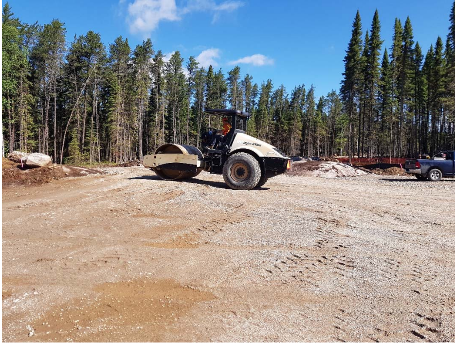
Photo 1: Facing north from the west side of the drill site. A vibratory roller was used to pack the final layer of subgrade material.
