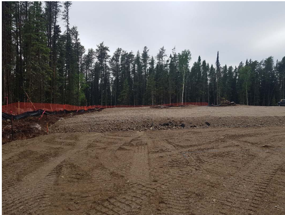
Photo 3: Facing west towards the elevated drill pad at IG_BH03. Perimeter silt and snow fencing can be observed to the left, and access road approach can be observed on the right side.
